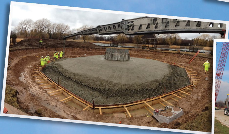
The foundation measures 100 feet in diameter, is over 10 feet deep, and contains nearly 700 yards of concrete.
